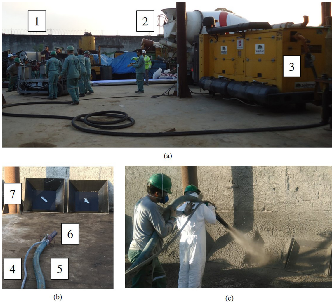
Fig. 4. Spraying process: organization of the process (a and b), concrete spraying process conducted by specialized nozzleman (c). Description of equipment: concrete spraying machine and accelerator pump (1), concrete mixer (2), air compressor (3), hose for accelerators (4), hose for concrete (5), nozzle (6), panels (7).
